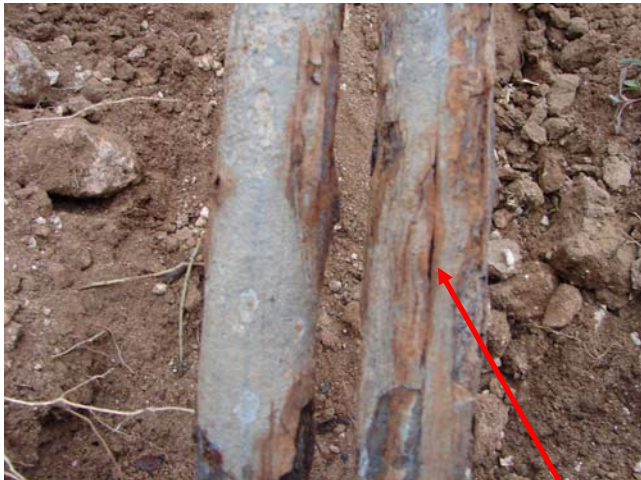
Close-up (2 Foot Below Ground Level) Note: Cracking of galvanized coating
