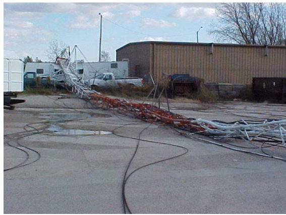
Morton, IL failed tower - 2001
