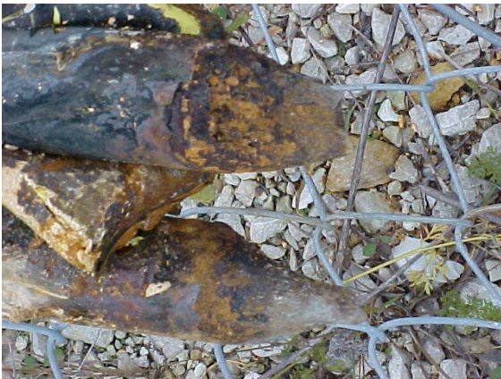
Failed dual anchor shaft – Morton, IL
