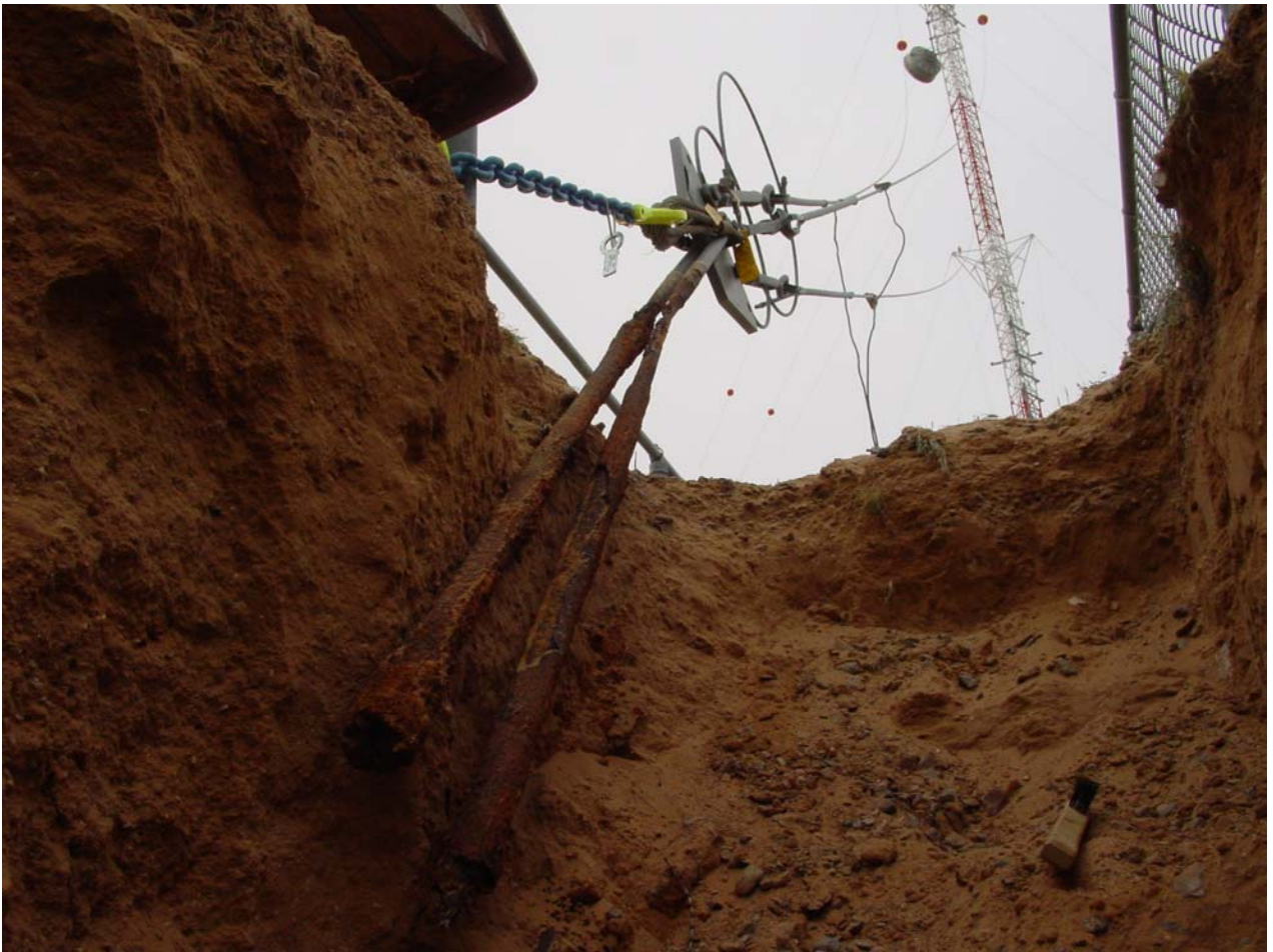
California 1/21/05 – Broken anchor showing slack guy wires
