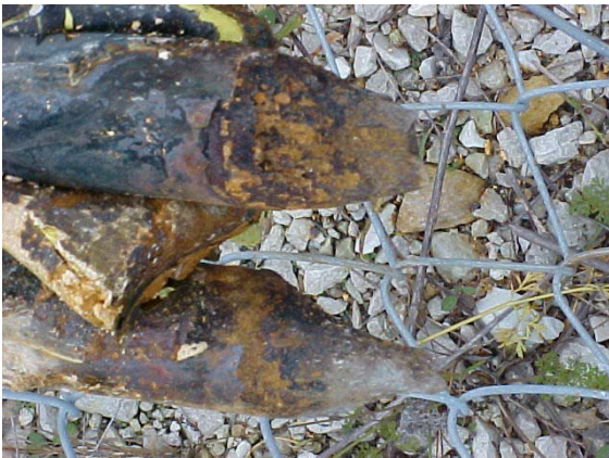
Failed dual anchor shaft – Morton, IL
