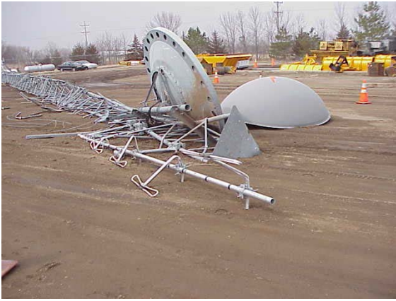
Mitchell, SD (installed 1989)
