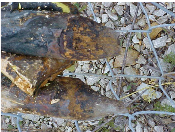
Failed dual anchor shaft – Morton, IL
