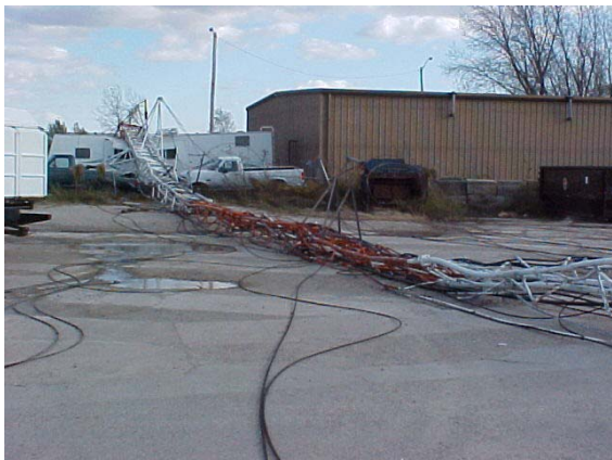
Morton, IL failed tower - 2001
