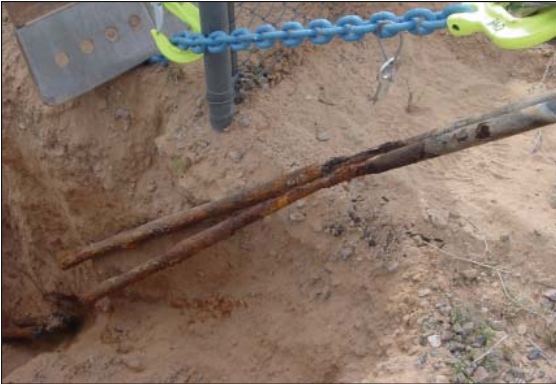
An anchor shaft break that occurred during inspection. The chain visible at the top of the photo was used to secure the guy to a piece of construction equipment as a safety precaution before excavation.
