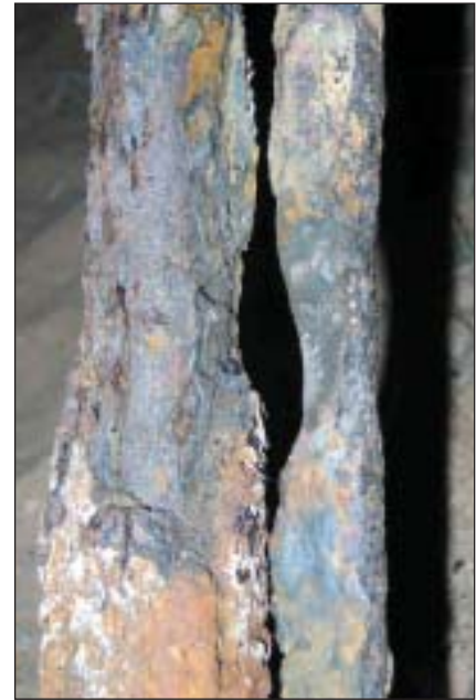
Corroded anchor shaft segments.
